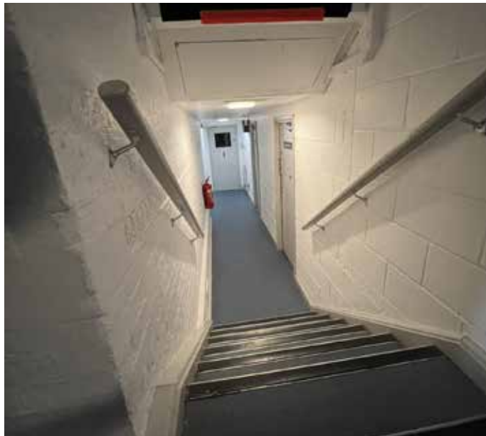
Level Access Issues
