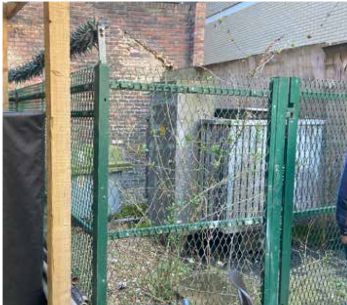
Limited Access to Substation
