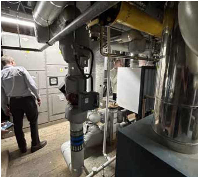
Limited Access to Plant Space
