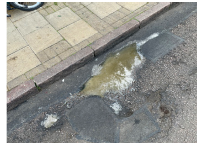
↑ Market Square: Leaking bin juice into the street creating an environmental and health hazard
