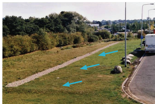
Filter strip leading to a filter drain. The filter strip removes silt and reduces the maintenance required for the filter drain, Hopwood services, M42
